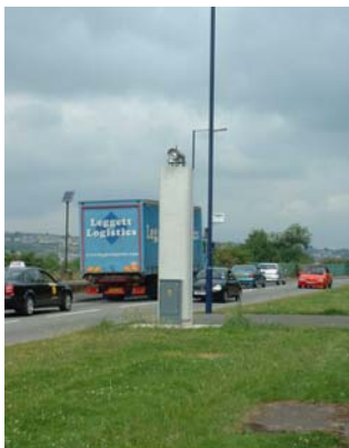
Photo 1 - St Thomas DOAS Transmitter
