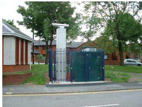
Photo 2 - St Thomas DOAS Receiver Station
